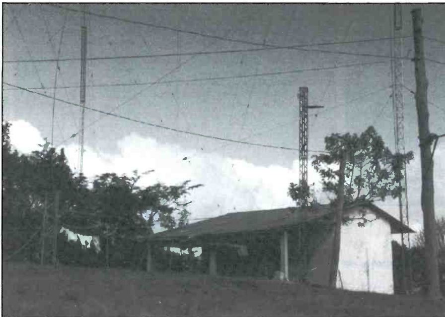
AWR-Guatemala's shortwave transmitter building antennas, in Cantos los Pilas.
